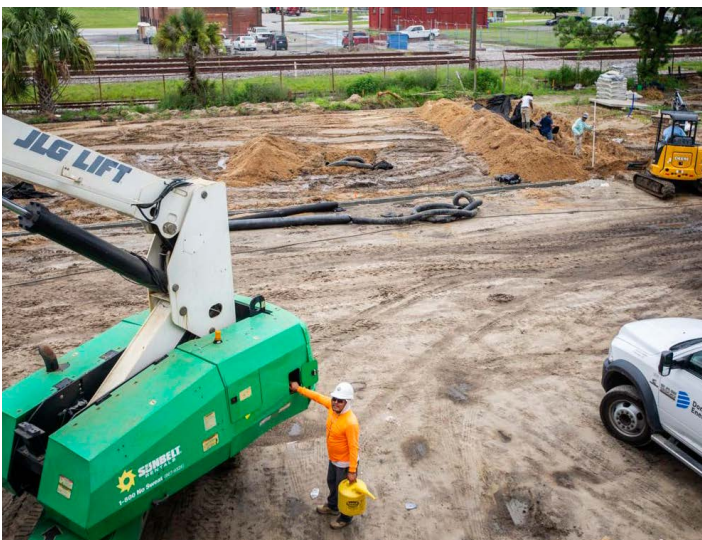
Construction continues on a ,1500-seat amphitheater at the 4-acre site of The Refinery at 1640 Meeting Street Road on Charleston’s upper peninsula in early July. The three-story building will include multiple office tenants and space for a restaurant. The project is set to be completed in October. Gavin McIntyre/Staff
