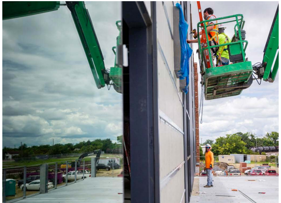
A construction crew works on the outside walls of The Refinery on Meeting Street Road in early July in Charleston. The three-story building will house offices and a restaurant and will include a ,1500-seat amphitheater in the back. Gavin McIntyre/Staff
