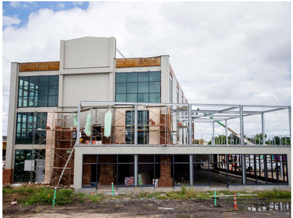
Construction continues on the 4-acre site of The Refinery, at 1640 Meeting Street Road in Charleston. The location was once part of the regional offices for Standard Oil Co. but will now be the home of an amphitheater, restaurant and office space. Gavin McIntyre/Staff
