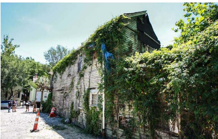
“This Old House” documented the restoration of this home on Bogard Street in the Elliottborough neighborhood. File/Kevin O’Connor/Provided
